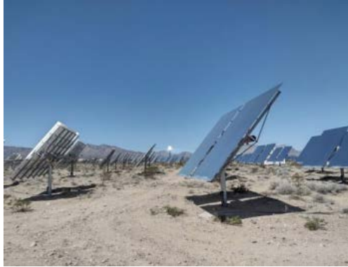
Figure 12. Illustration of solar field at Ivanpah power plant
